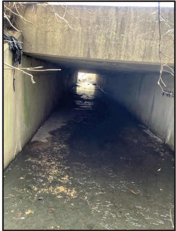
15. View of UNT 3 at existing box culvert inlet underneath Cypress Road, facing downstream east. 1/31/2024
