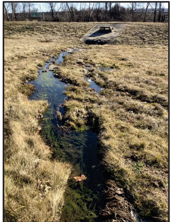
28. View of SF 7 draining from UNT 4 to detention basin inlet, facing south. 1/31/2024
