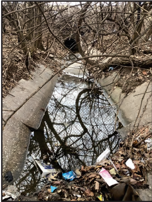
21. View of SF 5 and culvert outlet draining into UNT 3 – Concrete Portion, facing south. 1/31/2024
