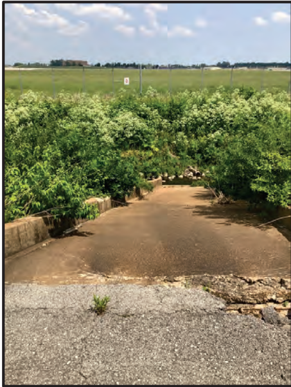
41. View of SF 2 draining into Coldwater Creek, facing north. 5/24/2023
