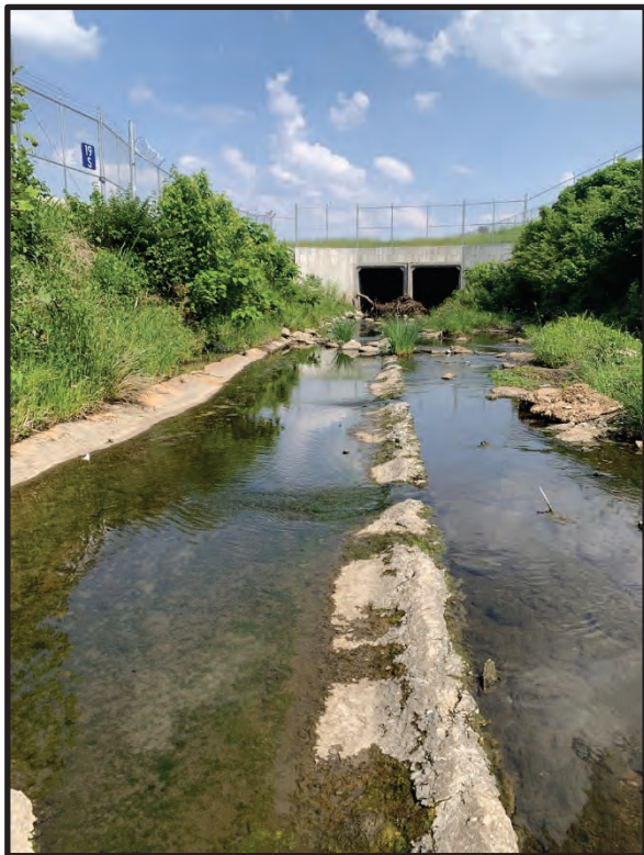
54. View of Coldwater Creek at existing box culvert inlets, facing downstream southeast. 5/23/2023
