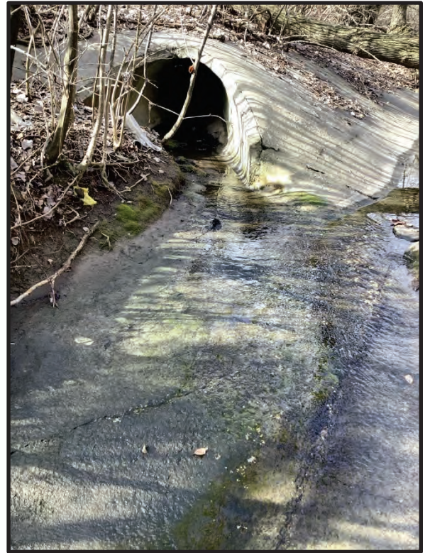
19. View of SF 6 and culvert outlet draining into UNT 3 – Concrete Portion, facing southwest. 1/31/2024
