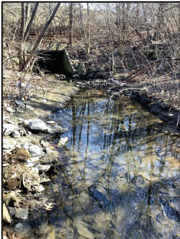
10. View of UNT 3 - Natural Portion at existing box culvert inlet, facing downstream east. 1/31/2024
