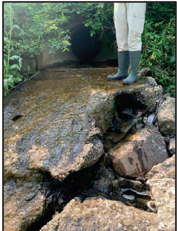
40. View of UNT 2 and culvert outlet draining into Coldwater Creek, facing upstream south. 5/24/2023
